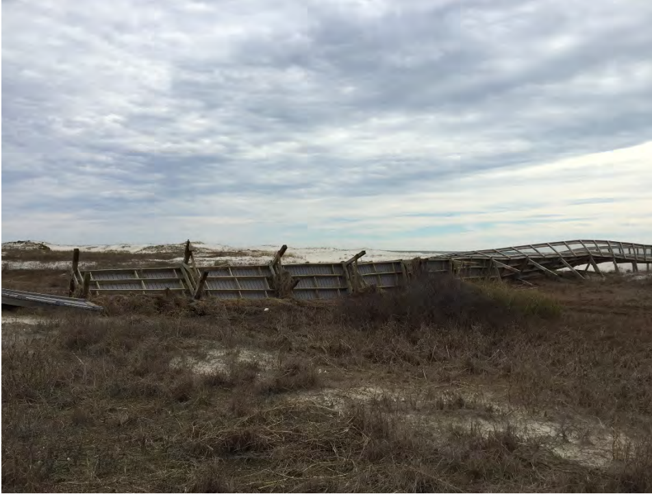
Figure 81. Beach crossover damaged by the storm in Zone SG-12.
