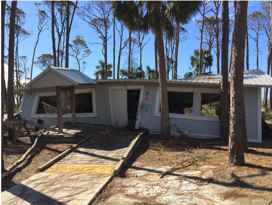
Figure 102. Significant damage to pavilion in Shady Pine campground.
